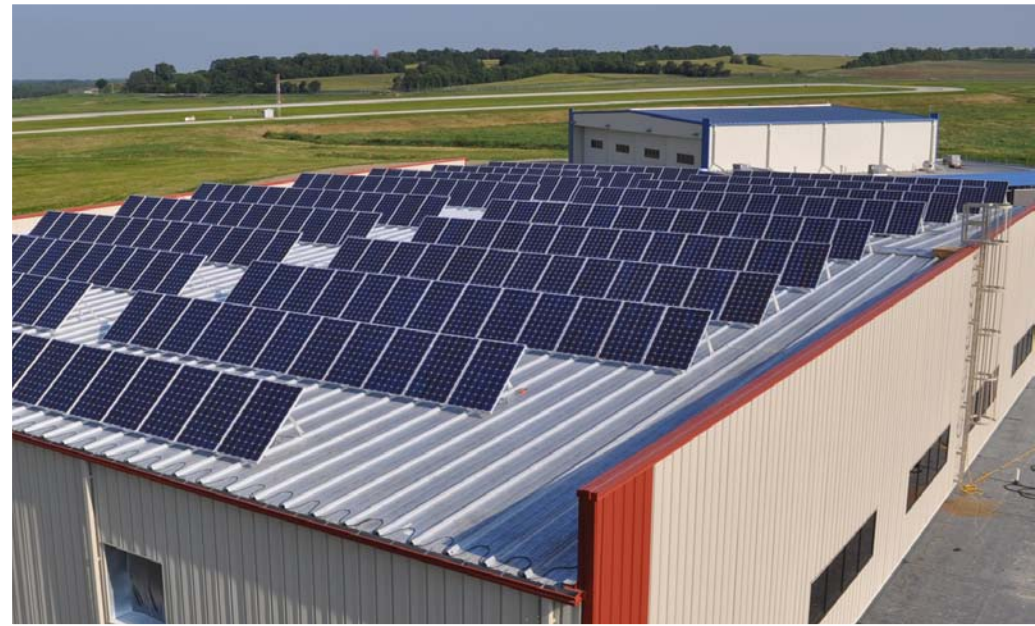
The solar array on the Promega Aviations Hangar is one of the largest statewide.
